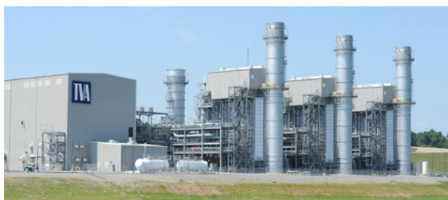
The Tennessee Valley Authority's Paradise Gas Plant in Drakesboro, KY opened in 2017.
